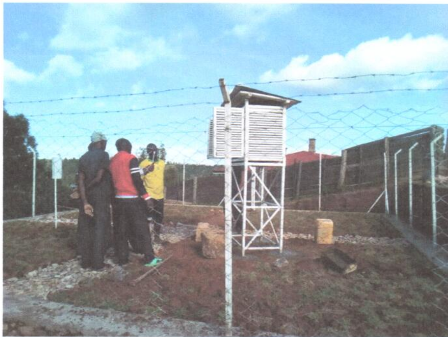
Kigeme relocated weather station
