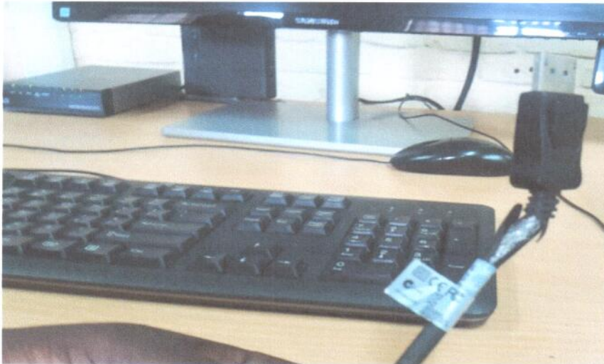
HDMI cable at is almost damaged at Meteo Rwanda Radar terminal site
